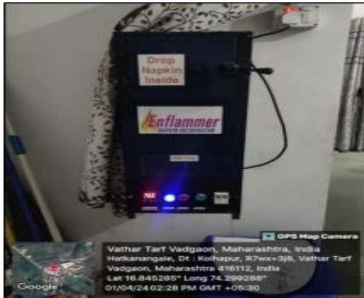
Fig 3: Sanitary Napkin Incinerator
