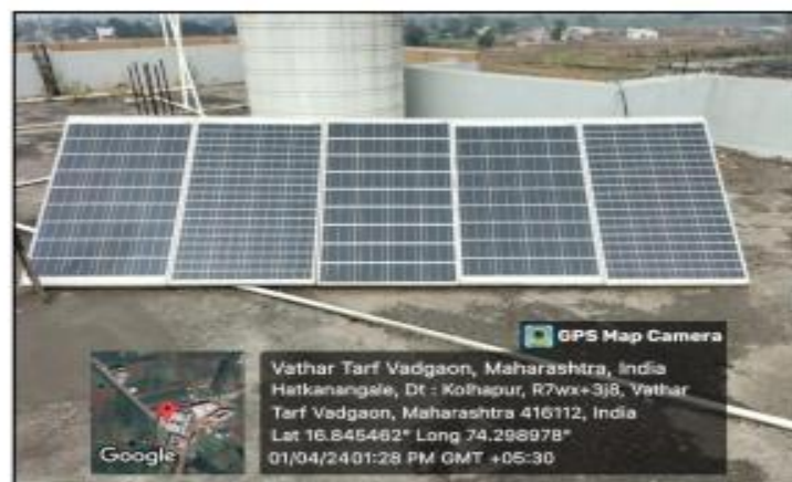
Fig 2: Solar panels at roof of college building
