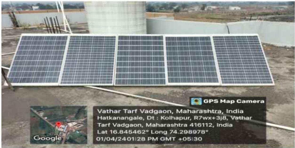
Solar Panels at roof of college building
